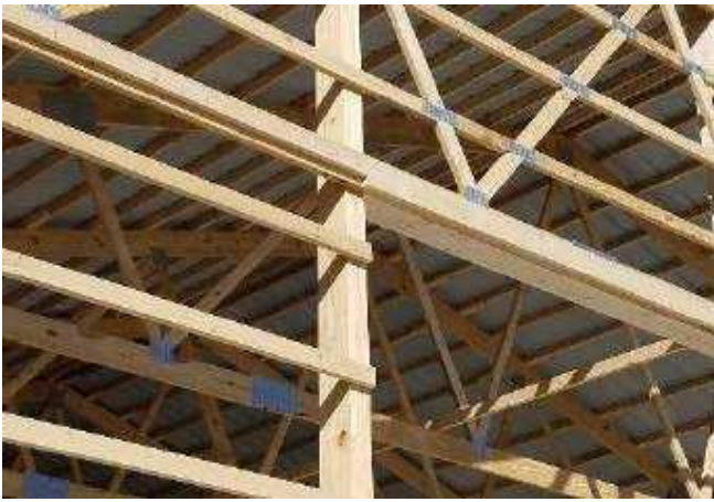
19. Track board. Ideal if 2x6 through opening & 2x4 beyond, door will work with whatever but critical dimension is 1 1/2" over framing plane where sheathing is fastened (over header)
