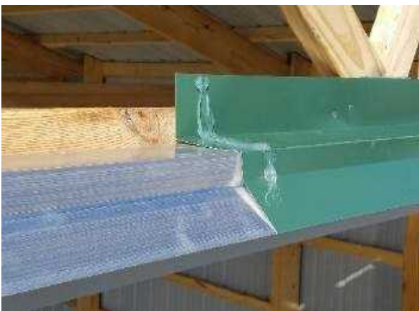
22. Install track cover; lock over weather guard & nail into header. Very crucial to caulk all laps and corners.
