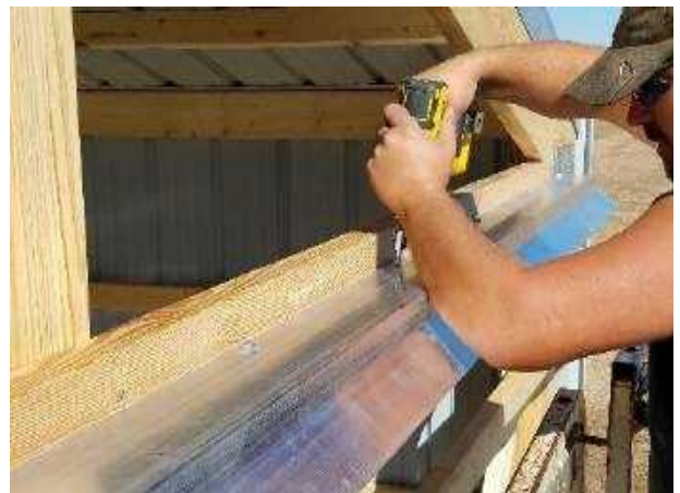
21a. Fasten track with lag bolts through pre-drilled holes with 5/16" x 3" lag bolts nail into header.
