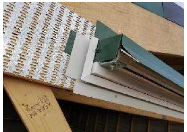
22a. Cut end of track so you can fold down to give it a better finished look. Do not fold down until doors are installed
