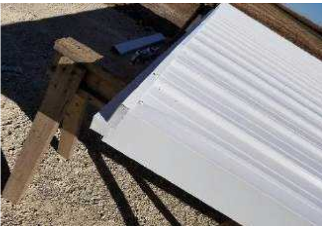
17. Fasten hat trim to top of C on back side & through every other rib on face. If trim is spliced, IT MUST BE CAULKED AT SPLICE.
